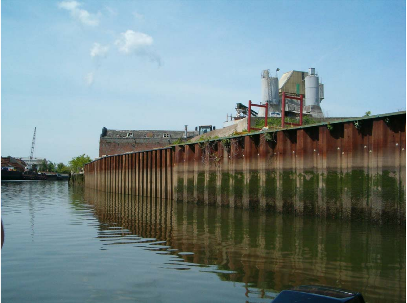
Repaired bulkhead on south side of Glen Cove Creek below Nassau Ready Mix and the old LiTungston plant (5/13/09) (photo by Carol DiPaolo)
