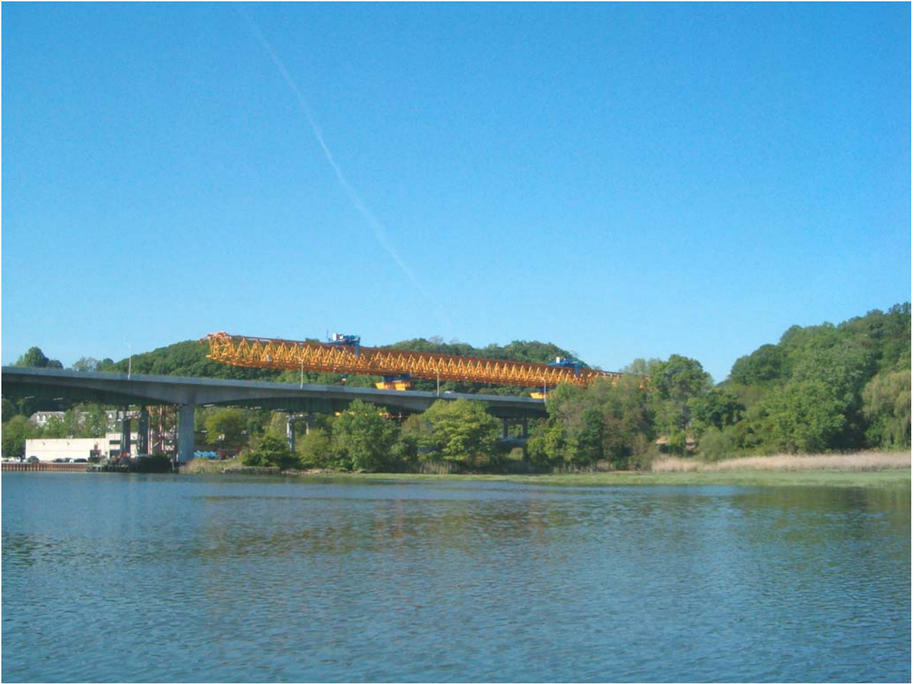
Gantry on western side of Roslyn viaduct to begin demolition and reconstruction of south side of viaduct (5/13/09)(photo by Carol DiPaolo)
