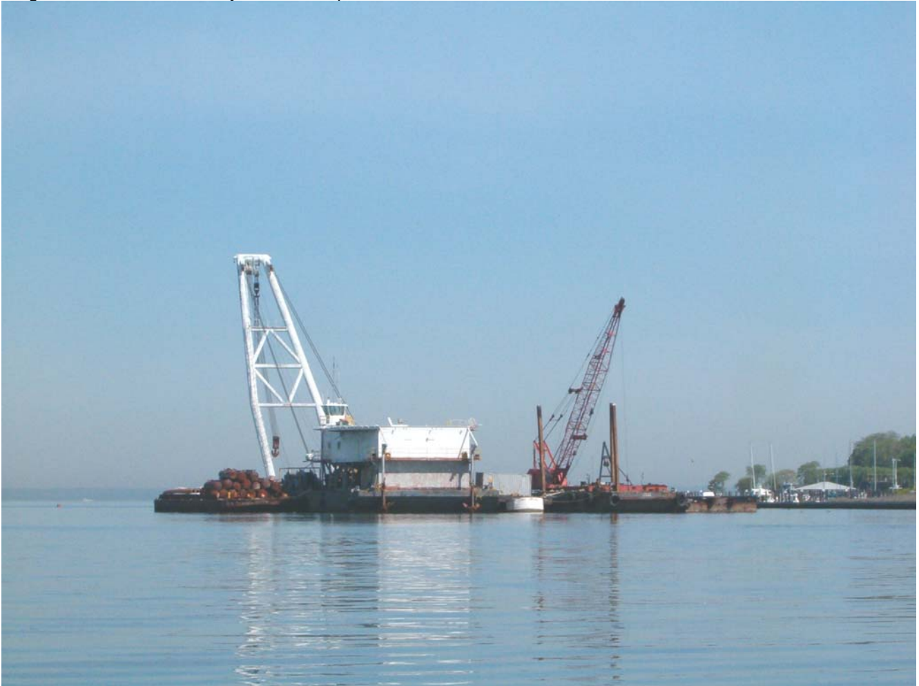
Gladsky cranes and barges off shore, north of power plant (5/20/09) (photo by Carol DiPaolo)
